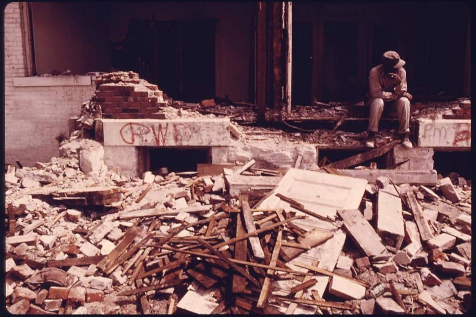
Demolition of Housing in Low Income Neighborhood -- Kenneth Palk, Kansas City, KS
